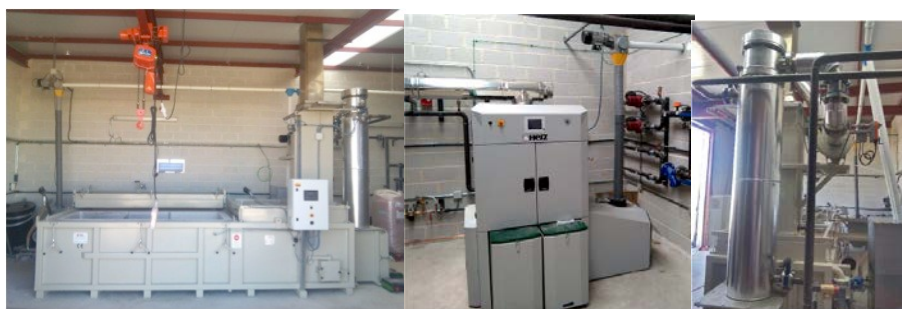
Figure 6 a,b,c. Centralized facilities with large on farm equipment in a pig farm (Spain) a) feeding equipment of biomass into incineration b) Biomass boiler; c) Heat recovery.
