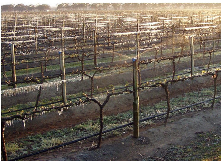
Figure 3 Example of Netafim Pulsar system installation.
